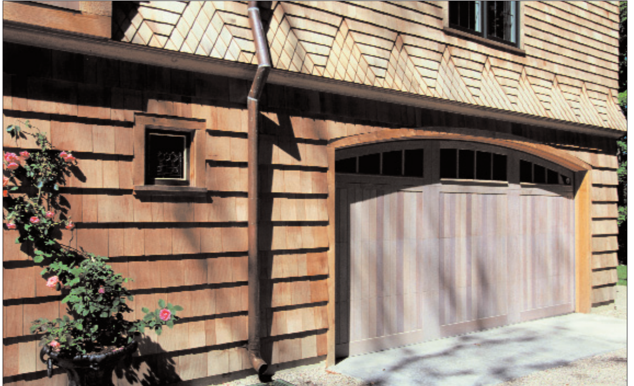
This close-up of the garage doors highlights the diamond-shaped detail in the shingles on the upper portion of the house. Bruce LaRose Custom Millwork made the doors. All photos: Carolyn L. Bates, Burlington, VT
